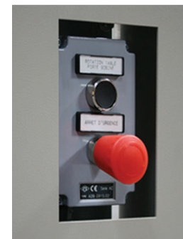
Detail of control panel
